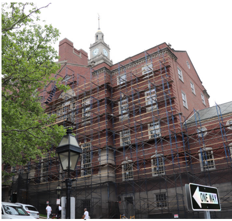
Brick work, masonry, and windows were restored and repaired at the Licht Judicial Complex, Providence.
